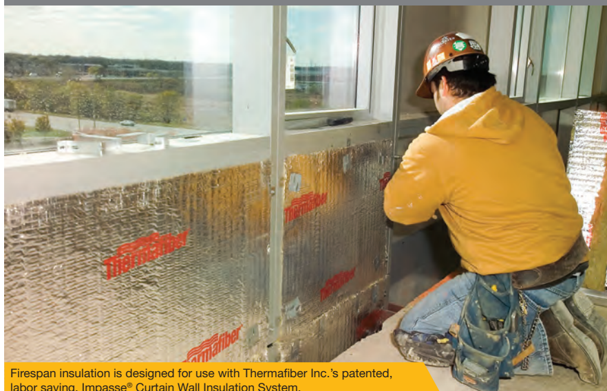
Thermafiber insulation provides the critical components of the perimeter fire containment system in the Trump International Hotel and Tower in Chicago.
