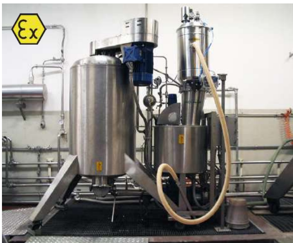
Perlite transport system, compressed air for ATEX 1-2 zone on a filtering unit in a distillery.
