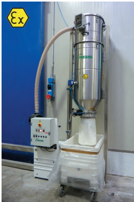
Pneumatic conveyors system for flour and processing residues in an industrial pizzeria. System realized in version ATEX for zone 22 powders.
