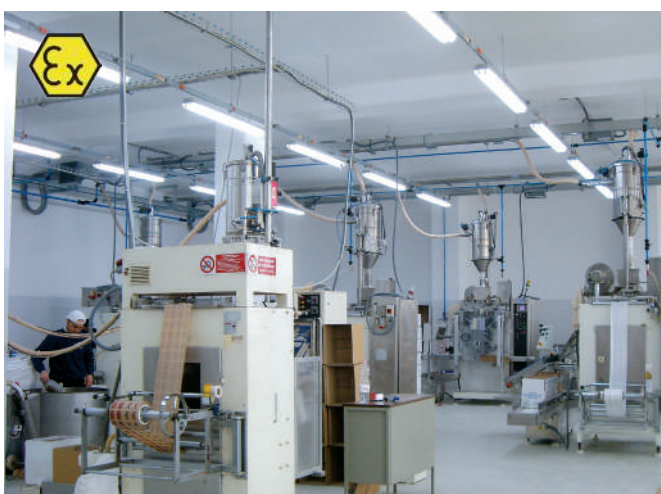
Pneumatic transport system on a total of 9 packaging machines with 4 big-bags removal in a sugar packaging industry. System realized in version ATEX for zone 22.
