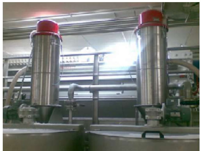
System consisting of two single-phase conveyors that load two tanks for the preparation of the fossil flour filtration compound.
