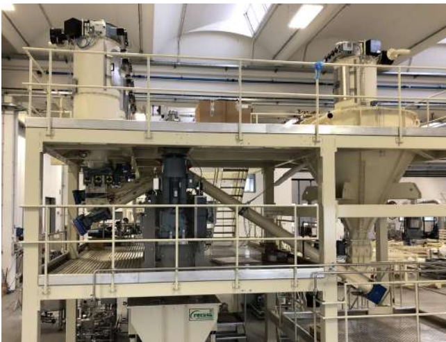
Pneumatic conveying system for tobacco powders, storage in silos and dosage on mixer.
