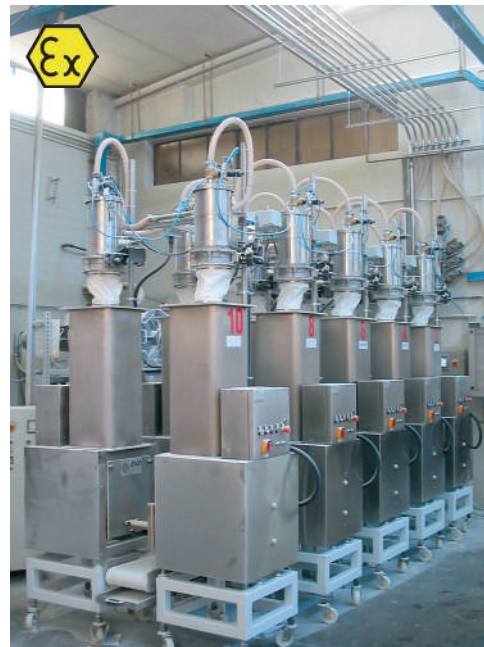
Conveyor and dosing plant with recipe management (10 products) in an industrial bakery. System realized in version ATEX for zone 22 powders.
