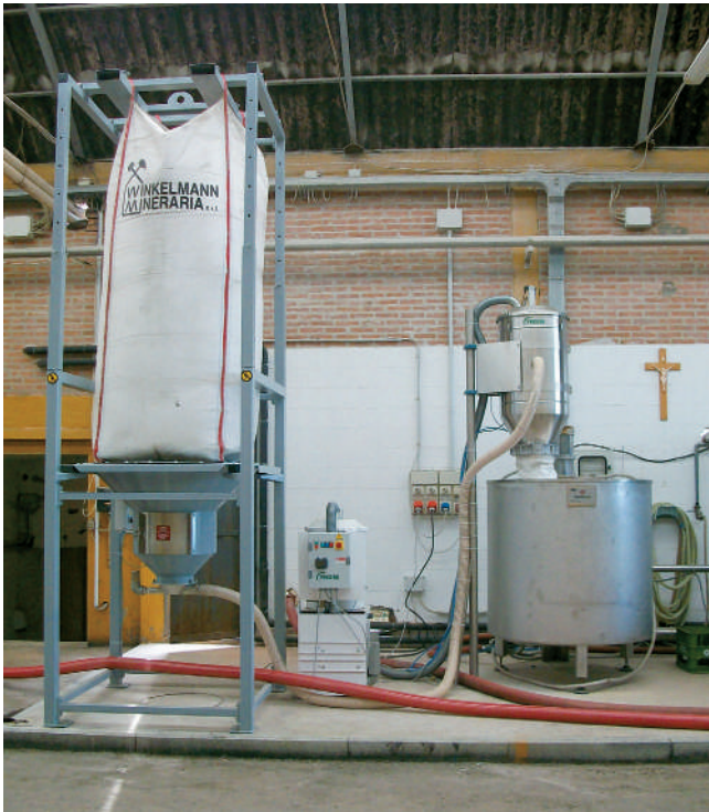
Fossil flour conveyor system with big-bags emptying system and transfer on filter in a cellar.
