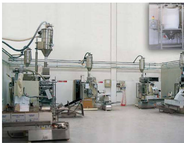
Loading hoppers for conveying of sugar.
