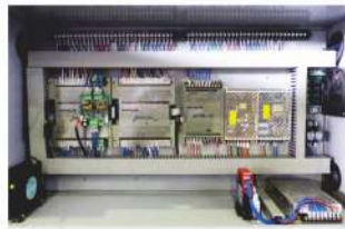
DC電氣箱 DC Electric Box
