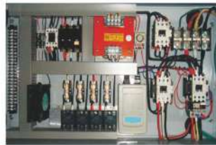
AC電氣箱 AC Electric Box
