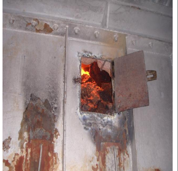
啓動後結塊滾到監視孔 After blowing
