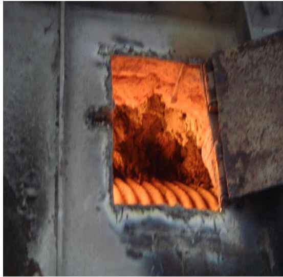
鍋爐內結塊 Clinker in the Boiler
